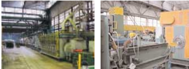
Furnace and polishing equipment in the Costa Volpino plant
